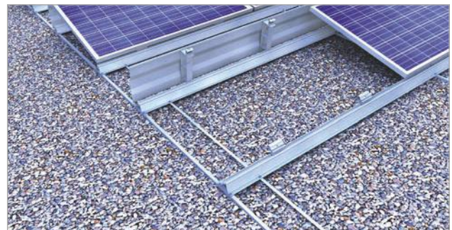
On gravel: south system I with gravel as ballast
